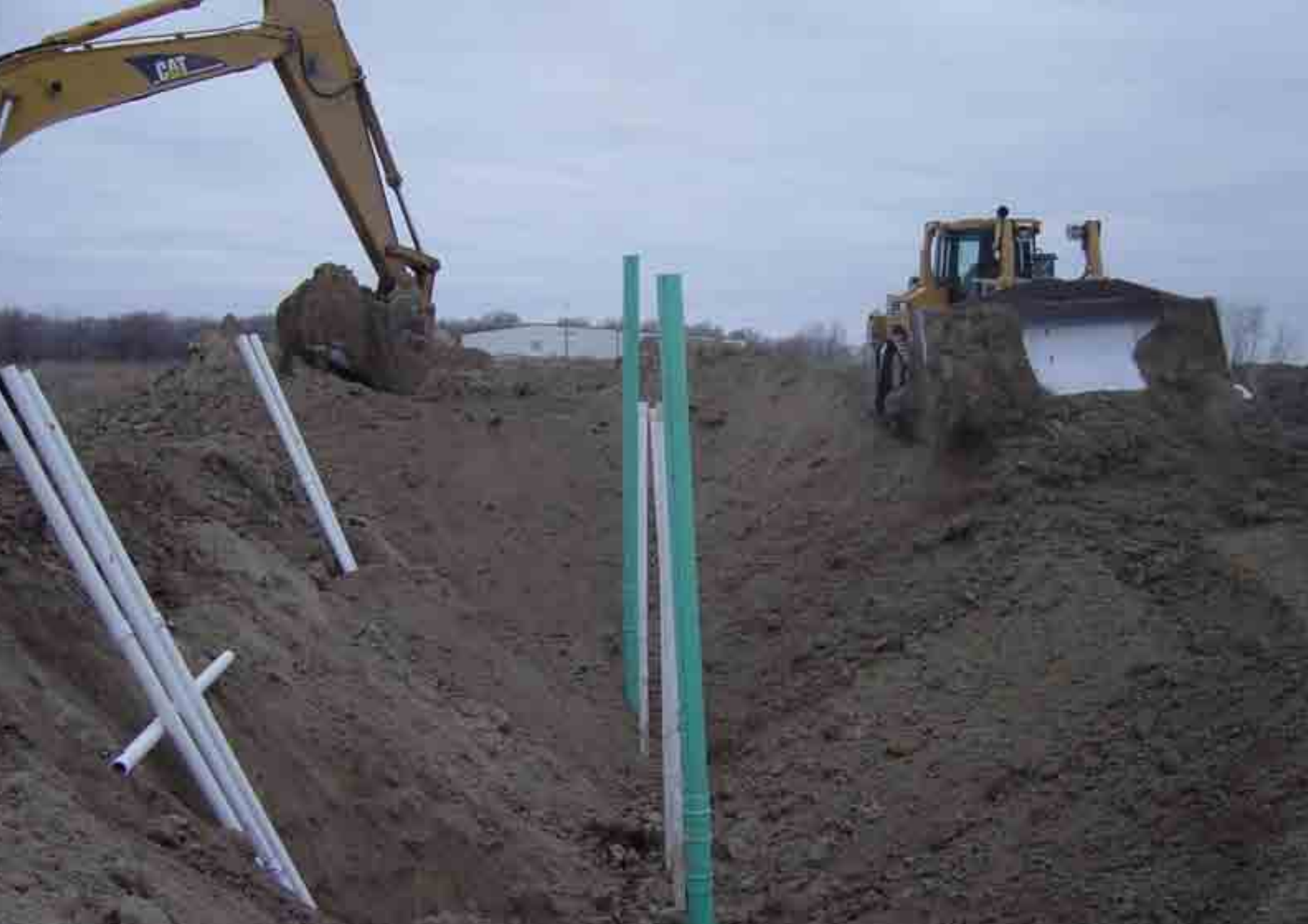
Backfilling above the PRB. The white pipes are 3-inch access tubes for coring
