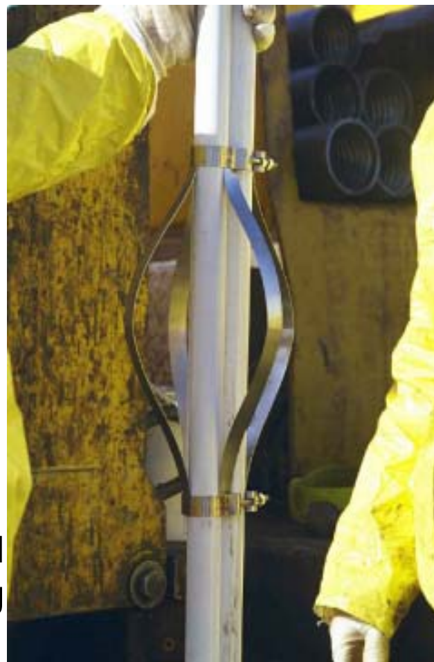
Centralized sampling pipe
